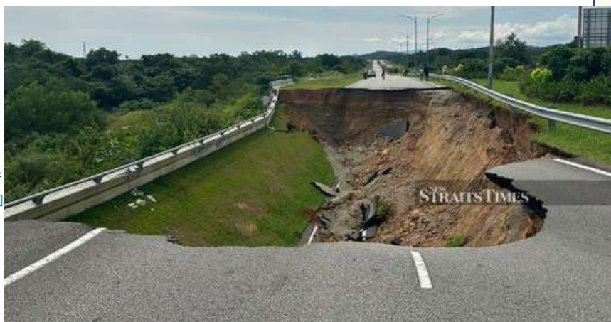
A collapsed 25m stretch of bridge [3b]
